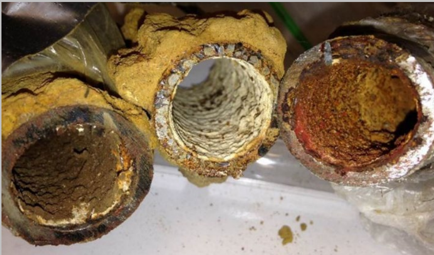
View into Flint drinking water pipes, showing various types of iron corrosion and rust. Min Tang and Kelsey Jeper
